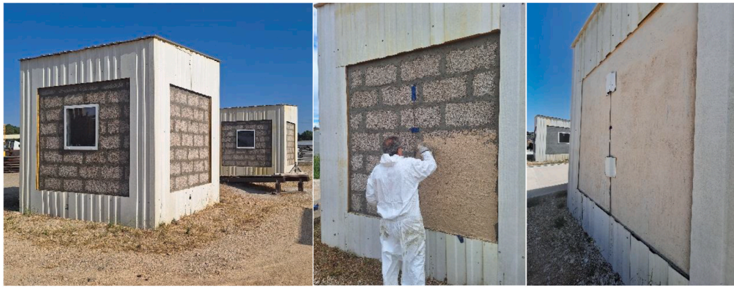
Fig. 3. Pilot-scale mock-ups with hempcrete baseline, illustrating the construction stages: application of the external rendering system on the hempcrete substrate and the final appearance of the hardened mortar layer on the external façade.
